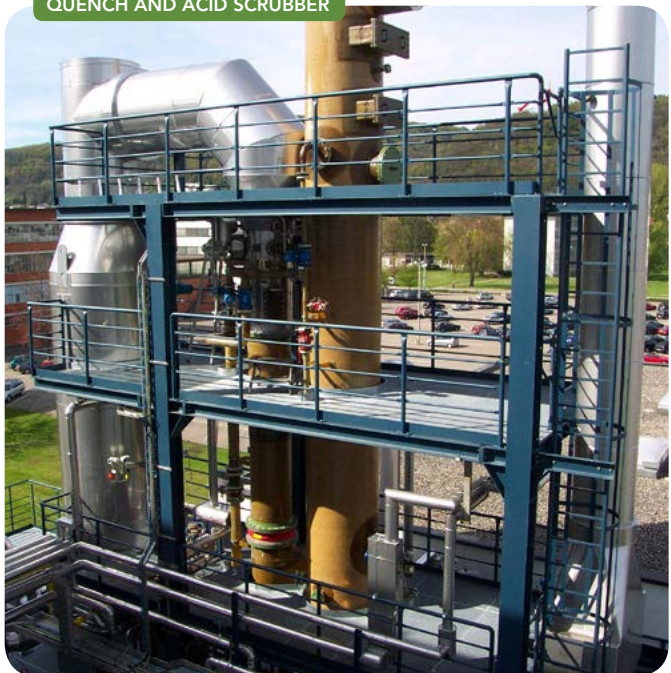
Figure 3. After exiting the economizer, the flue gas is directed to a quench and acid scrubber, much like this one.
